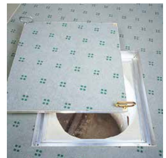
built-in in the office (cleaning shaft), lined with carpet
